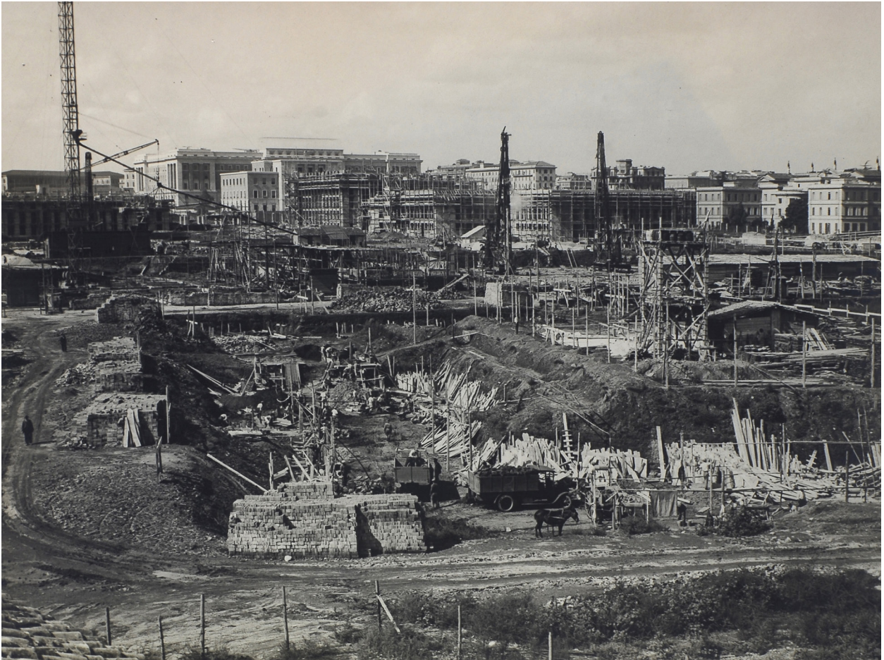
Fig. 6. Excavations for the foundations of the Sapienza Campus buildings, July 1933. (Author: unknown. Source: Sapienza Historical Archive).
